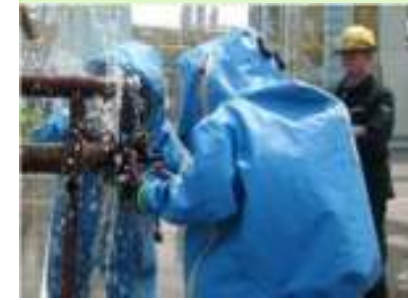
泄漏处置 Deposition of leakage
